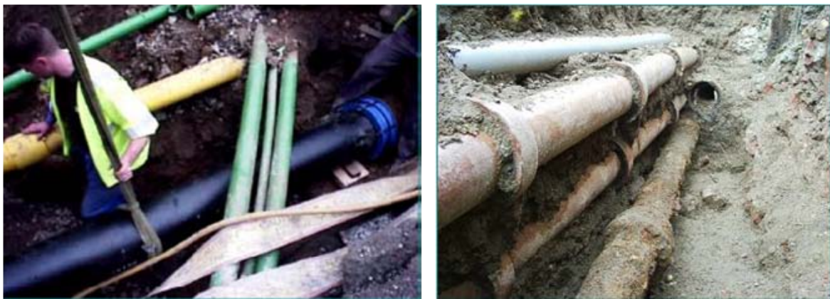
Figure 1: A typical tangle of pipes and cables under our city streets that can result in expensive third party damage
